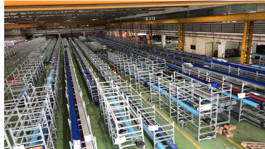
Modular M&E services installation
